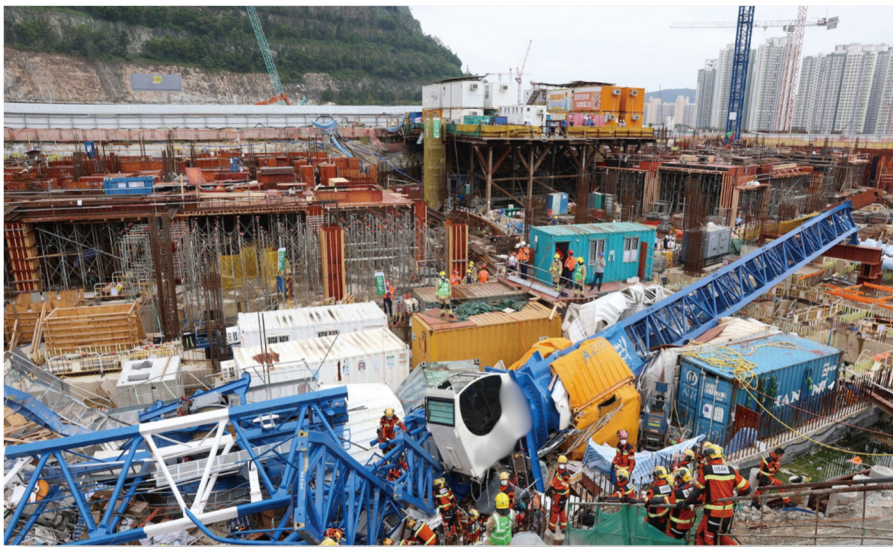
Figure 11: A fatal work accident at a construction site at Anderson Road, Sau Mau Ping in 2022
