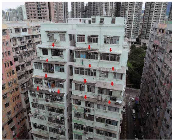
Figures 6 and 7: “Street shadow building” (the arrows in red are pointing at UBWs, which are canopies erected at places that have been set back)
