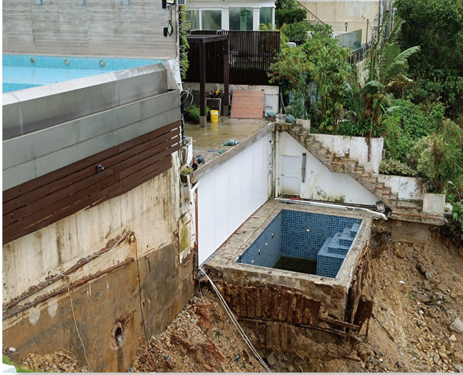
Figure 8: Example of “serious UBWs” (last year's rainstorm revealed some large-scale UBWs in certain houses, such as the unauthorised swimming pool shown in the photo below, with landslides occurring on the surrounding slope)
